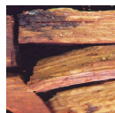
Yellow dry slaty rot - YDS Characterised by wood that superficially appears intact, but is dry, lightweight, brittle, and inclined to break along the growth rings. The grain of the wood often has a sheen. It occurs mostly in the outer heartwood.
