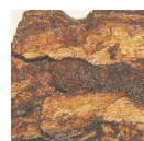
Dark borer wood - DBW Has a fibrous or spongy red-brown rot, which is rather moist and contains galleries of termites or other borers.
