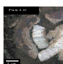
Pale stringy rot - PSR Composed of continuous long, spongy, wool-like, bleached-white fibres. Crimson to dark brown solid wood is always found adjacent. Often associated with the outer heartwood, and sometimes in contact with the log surface, though columns occur within inner heartwood.
