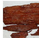
Dark blocky fibrous rot - DBF Has a distinctive red-brown colour. Breaks into irregular blocks, and maintains a soft, fibrous, texture. Even when the wood is hard, the fibres can be teased apart. In more decomposed wood, the fibres are moist and soft, giving a spongy texture.
